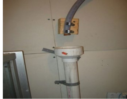
Softener discharge drain line with air gap
